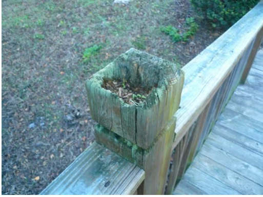
Deteriorated wood on decorative rails and footbridge
